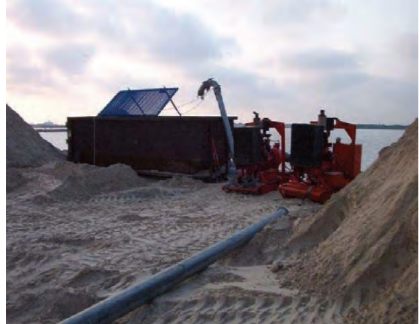
Slurry Pumps at the Ready
